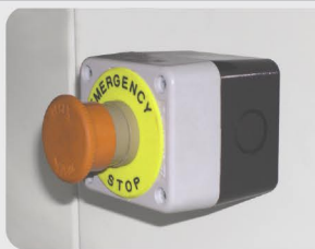
後部緊急開關 (後面收料人員, 可控制機械而減少不必要之損失) Emergency switch on the machines rear. (the emergency to stop working decision depend on rear operator. It can decrease lose when improper control.)
